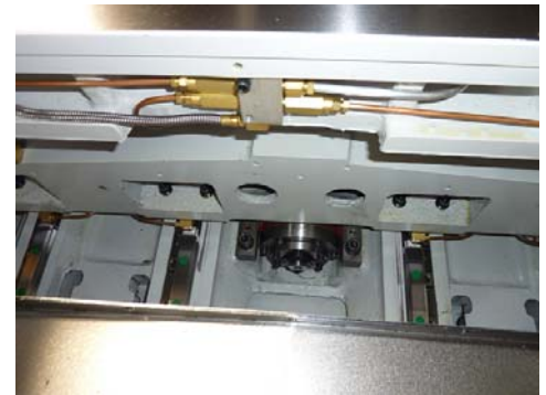
the ballscrews and linear ways are lubricated automatically by timer controlled oil injection
